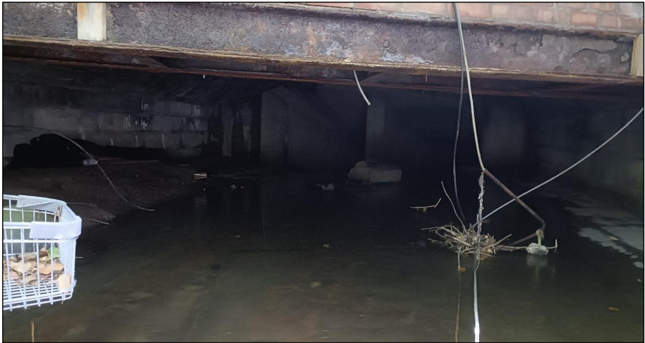
Figure 5-15: Carrickmines Stream N11 culvert displaying anthropogenic disturbance and sub-optimal Otter commuting
