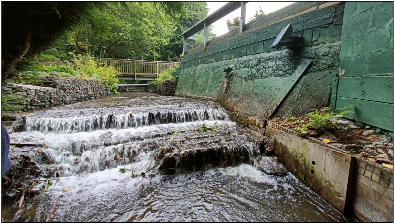
Figure 5-16: IFI-confirmed fish migration barrier along the Brides Glen Stream along Cherrywood Road
